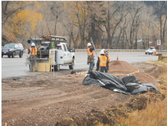
Construction workers build a temporary bus shelter in front of Basalt Realty, just upvalley from the current bus stop.
